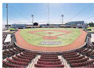
A baseball ground is being repurposed into a cricket facility after MLC acquired a long-term lease.
