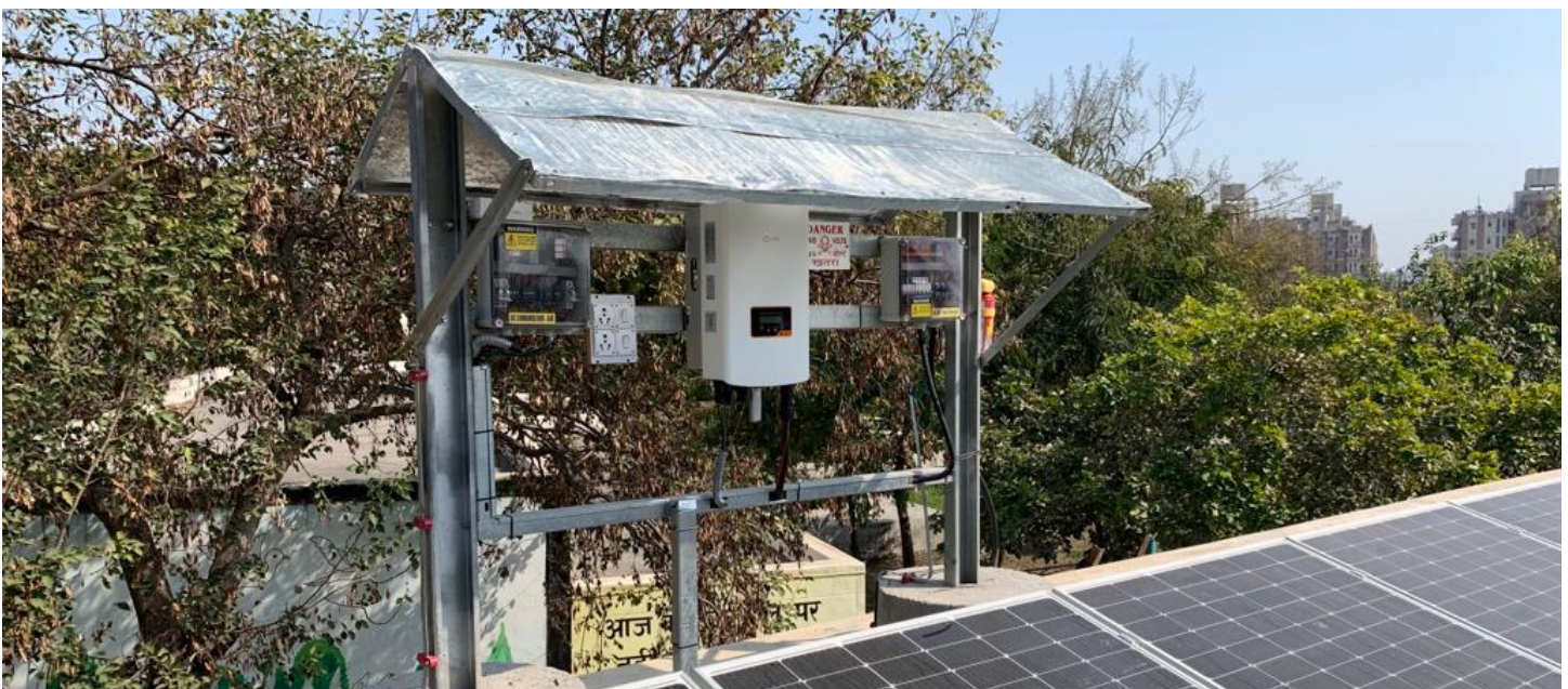
A solar power plant at a school in Gurugram
